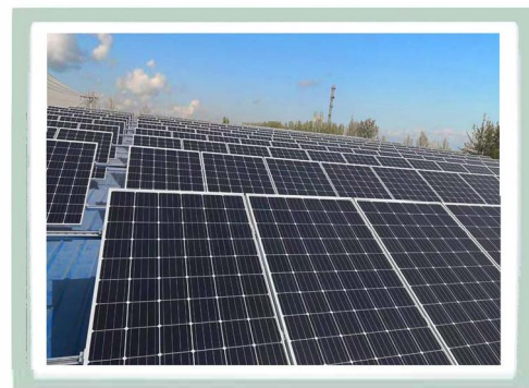
120kw solar power plant
