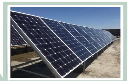
50kw solar power plant
