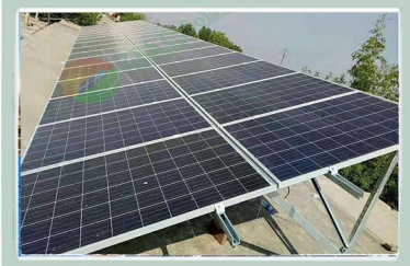
8kw solar power plant
