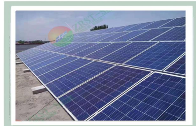
30kw solar power plant
