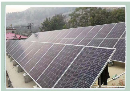
8kw solar power plant
