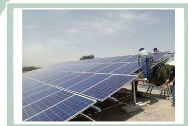
15kw solar power plant
