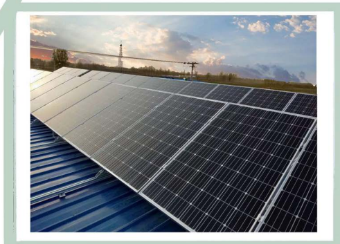
30kw solar power plant
