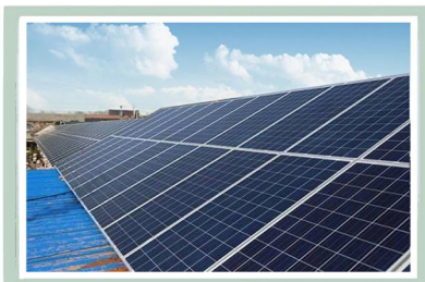
25kw solar power plant
