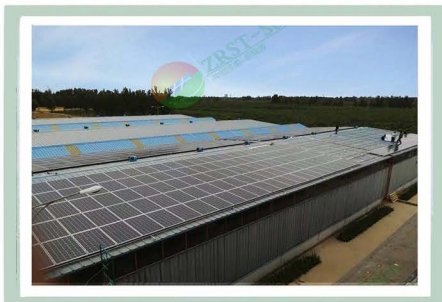
150kw industry solar power plant
